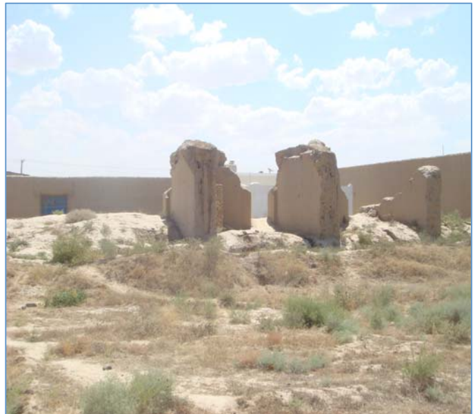
An extensively damaged premises of a Justice Institution recommended for Rehabilitation
