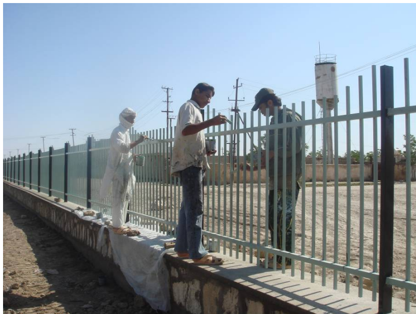
Construction of boundary wall, Jowajan province, Upgrading of Nine Vocational Training Center
